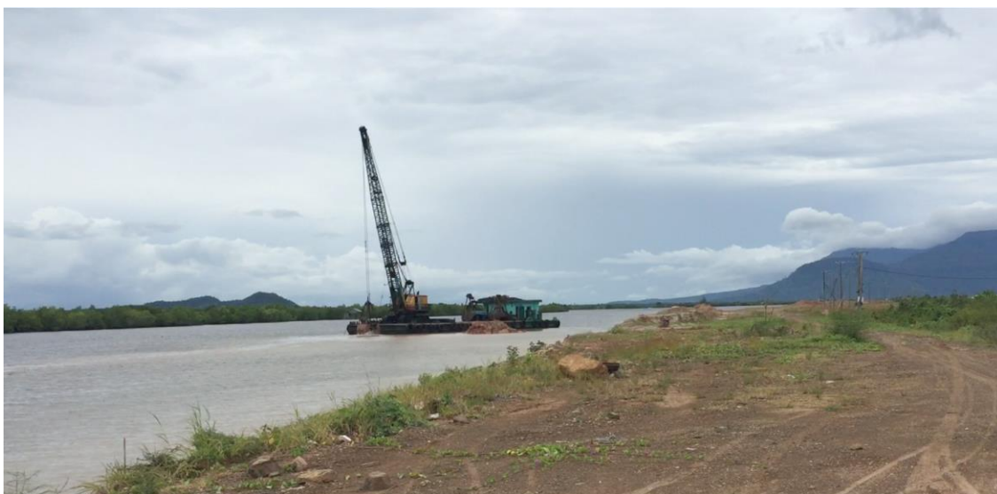
Figure 11: Digging soil next to the proposed Kampot pier location. Koh Samao is visible on the left.
