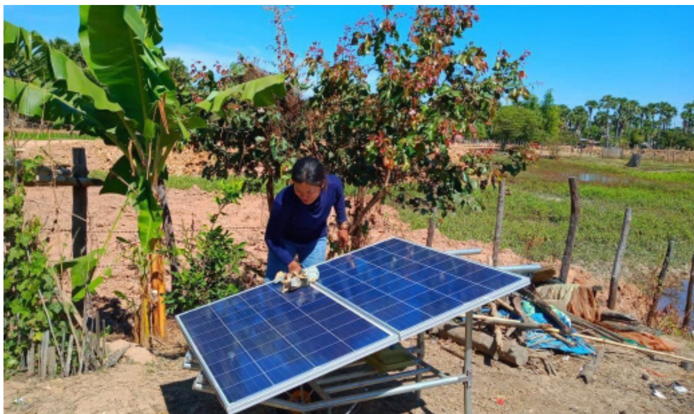
Sreymich is cleaning the solar water pump after used it.
